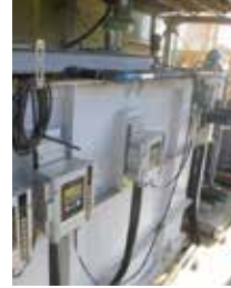
pH neutralization facility
