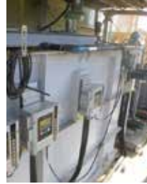
pH neutralization facility
