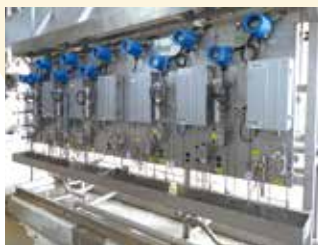
Boiler sampling system installed at a biomass power plant
